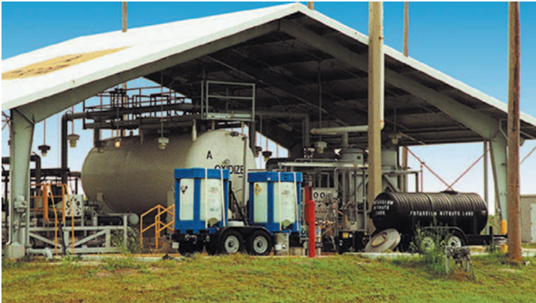
The Nitrogen Oxide Waste Conversion Scrubber installed at the oxidizer farm on Launch Complex 39A at Kennedy Space Center.
