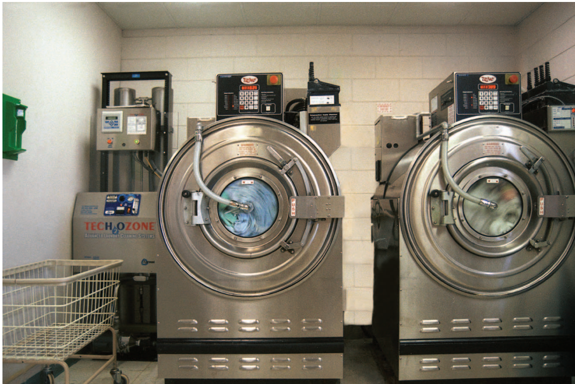
This version of the commercial laundry system shows the ozone generator mounted beside the laundry machines with the unit controllers mounted on top of the washers.
