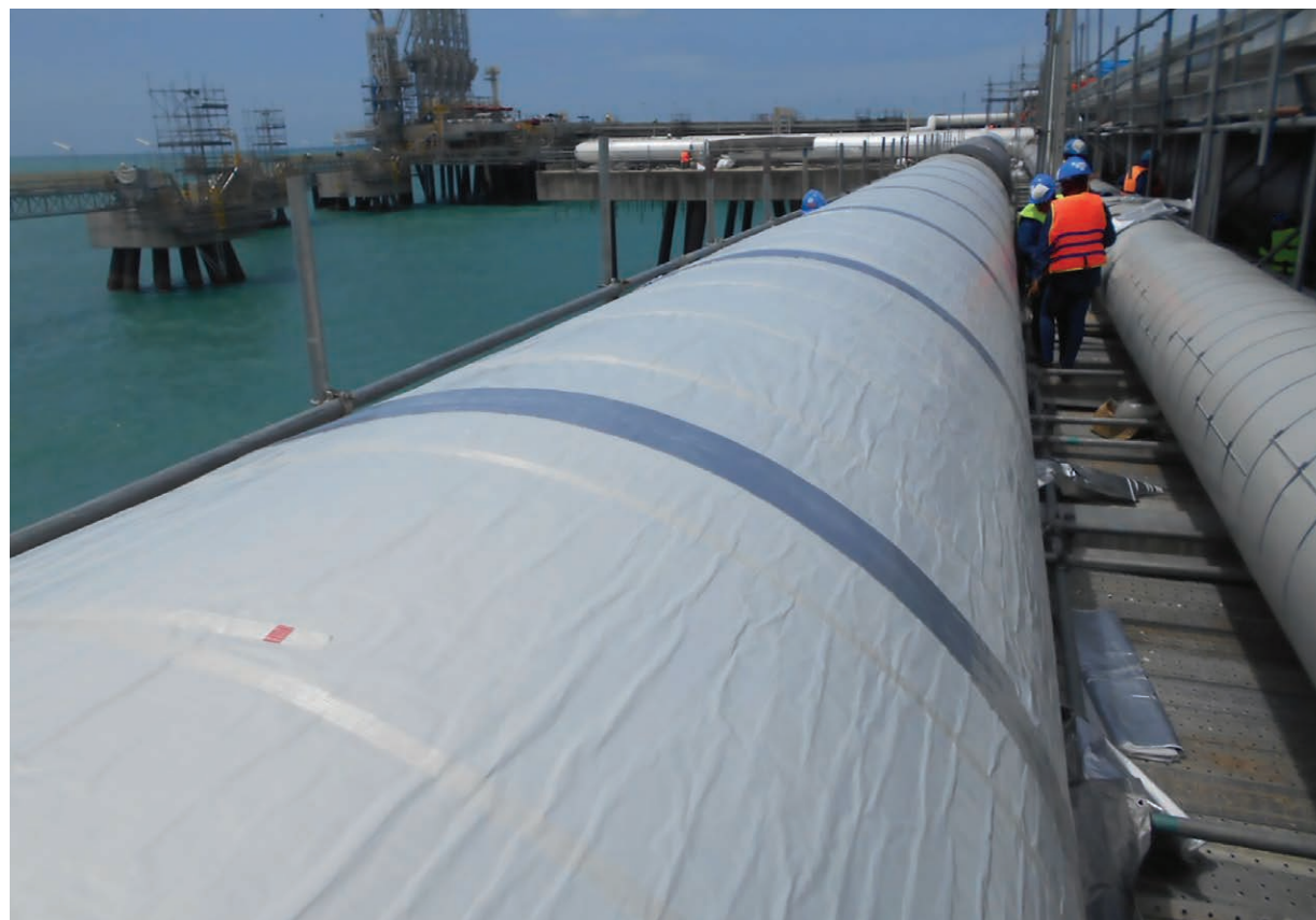
In the spring of 2019, Aspen Aerogels won a $40 million contract to insulate pipelines at this liquid natural gas receiving terminal in Thailand with its Cryogel Z insulation.
