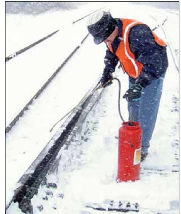
Railroads use Ice Free Switch, incorporating NASA technology, to stop water from becoming ice on train track switches. This helps to maintain train service during winter weather events.
